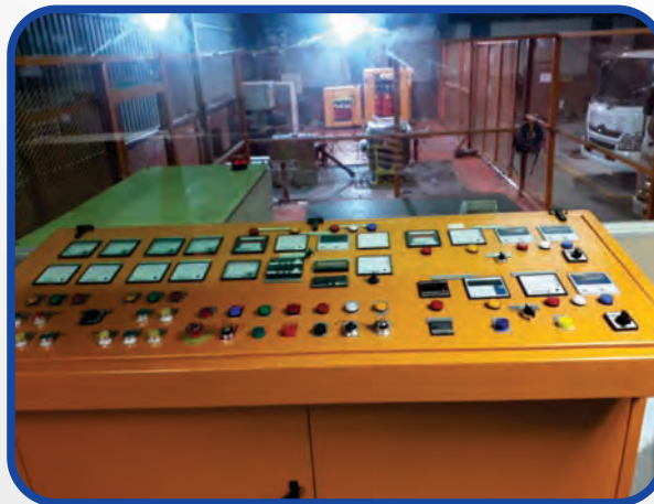
11 KV Test Facility
